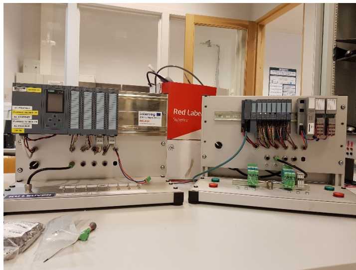
Figure 21: Small demonstrator set-up with PLC (left) connected to remote I/O (left), controlling electricity users (green modules before remote I/O).
