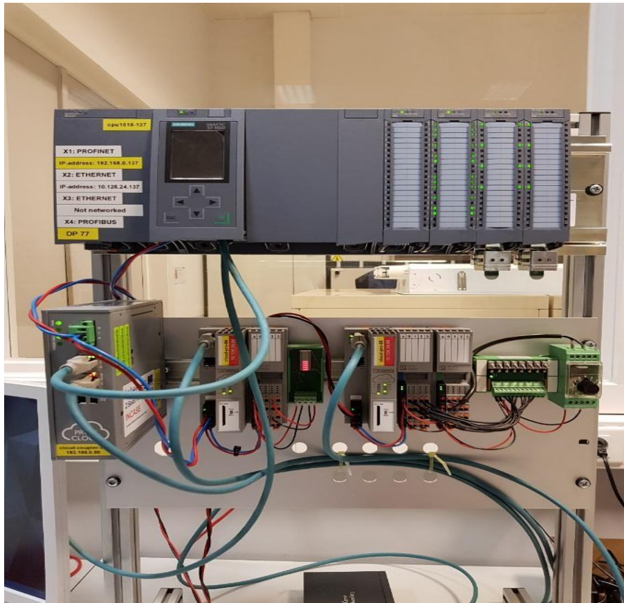
Figure 12: KUL local demonstrator with Siemens PLC
