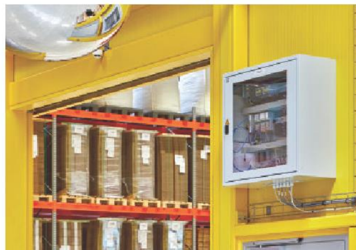
The AXC Cloud-Pro controller and the aligned I/O modules capture data from multiple temperature sensors that are distributed throughout the storage rooms.
